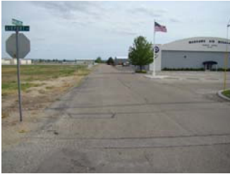
Poor pavement section on Municipal Drive
